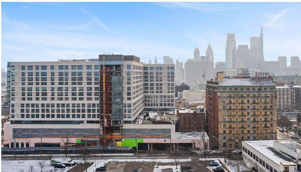
This photo, taken shortly before Christmas, shows some exterior work remaining on the Fairmount Avenue side of the building, where the main entrance will be located.
